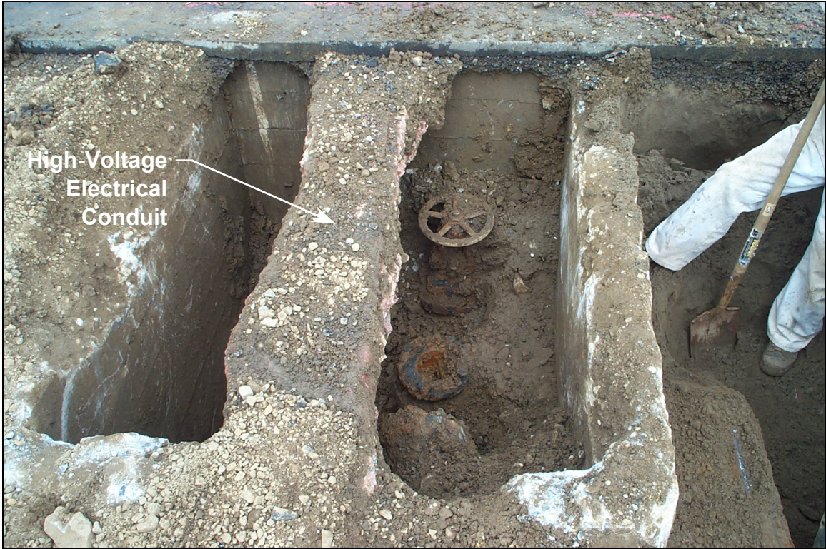
Photograph 1 - Concrete vault at EX-1 containing 6-inch-diameter piping and gate valves (view to north).
