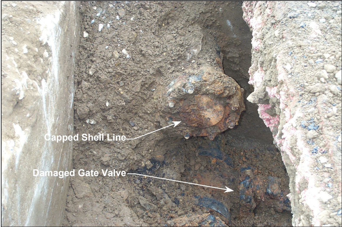
Photograph 3 - Close-up of capped Shell bulk plant supply line and Niemi/Mobil bulk plant supply line with damaged gate valve.
