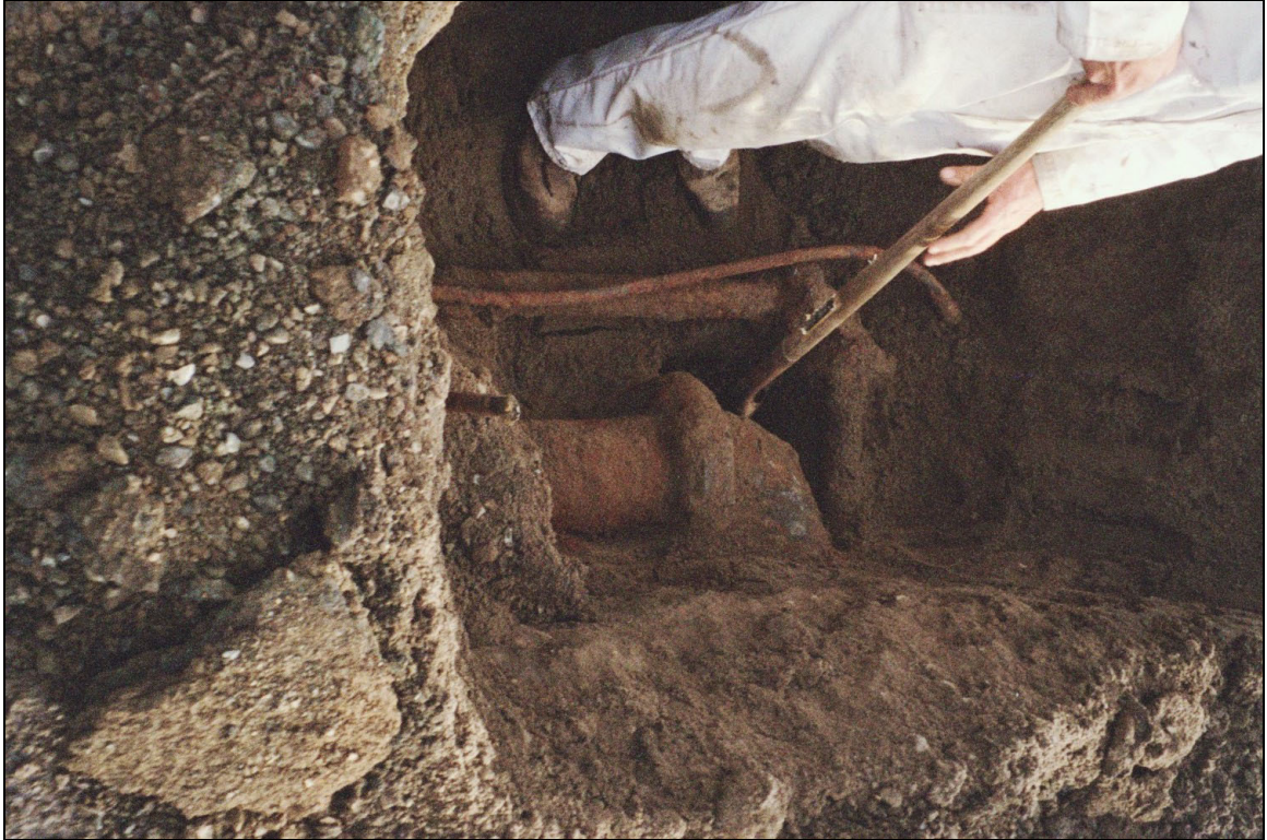
Photograph 5 - EX-3 location showing one 3-inch-diameter product line and the 6-inch-diameter product line with 90° flange joints.
