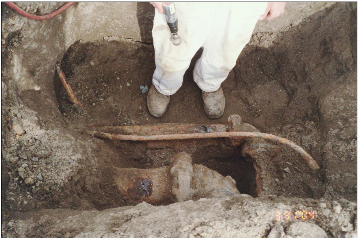
Photograph 6 - EX-3 location showing one 3-inch-diameter product line, the 6-inch-diameter product line with 90° flange joints, and an abandoned electrical conduit.
